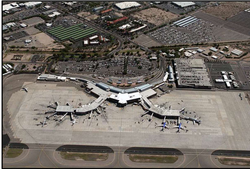
Figure 4: Project in progress – Tucson Airport application of the ceramic based thermal deflection paint [7]
